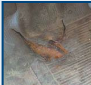
Excessive wear to floor coverings
