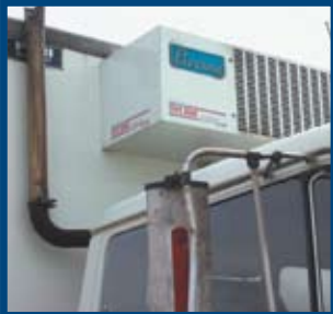
Broken, damaged exhaust stacks and missing rain caps
