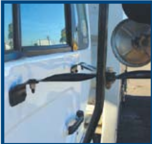
Any damage to mirror glass surround, framework or support
