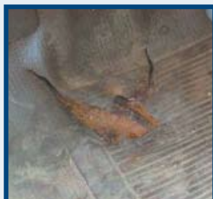
Excessive wear to floor coverings
