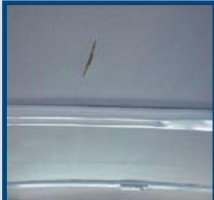
Damaged roof lining
