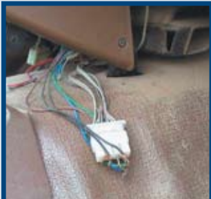
Untidy holes and wiring where after-market fitting has been removed
