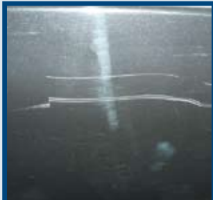
Isolated scratches over 20mm in length which penetrate to metal or primer
